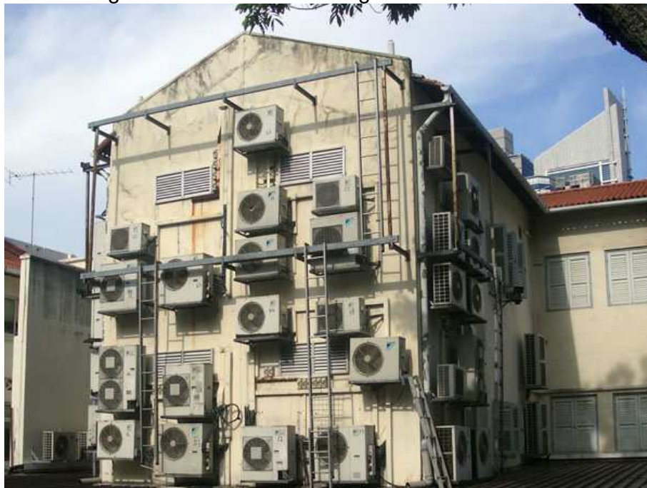
Fig. 22: Air conditioning systems for optimizing the sensing (onlineheld.de)
